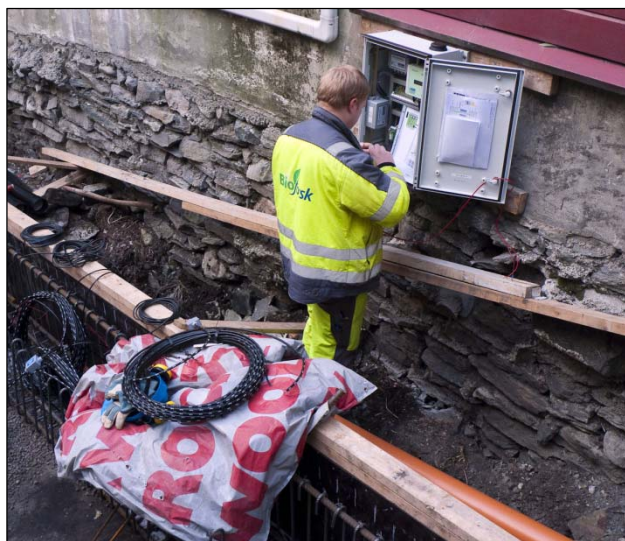
Figure 2. A waterproof cabinet for the automatic logger from SEBA Hydrometrie GmbH was installed on the wall close to the site.
