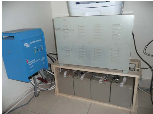
This arrangement provides enough power for 3 to 5 hours depending on the number of computers in use.
