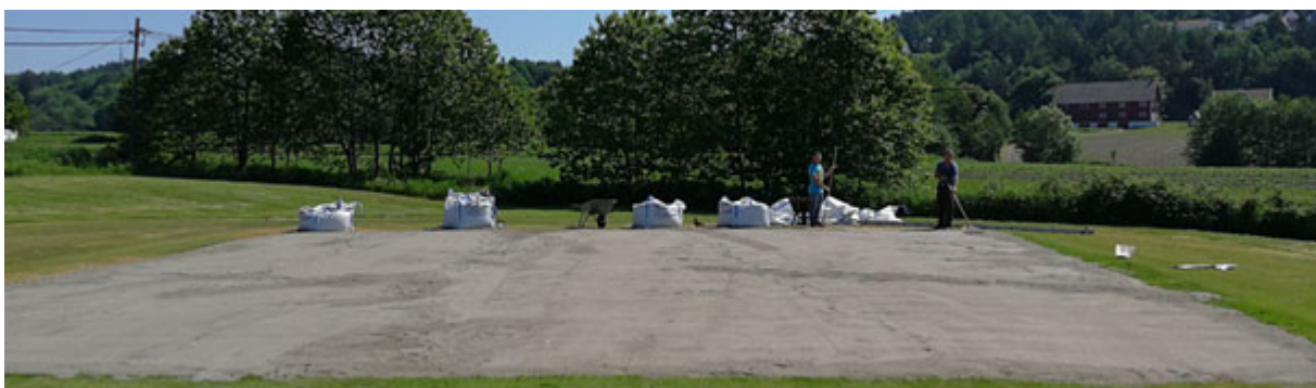
Figure 2. Replacing of 3-cm upper layer with new 12% peat growth media at Landvik on 30 May 2018.
