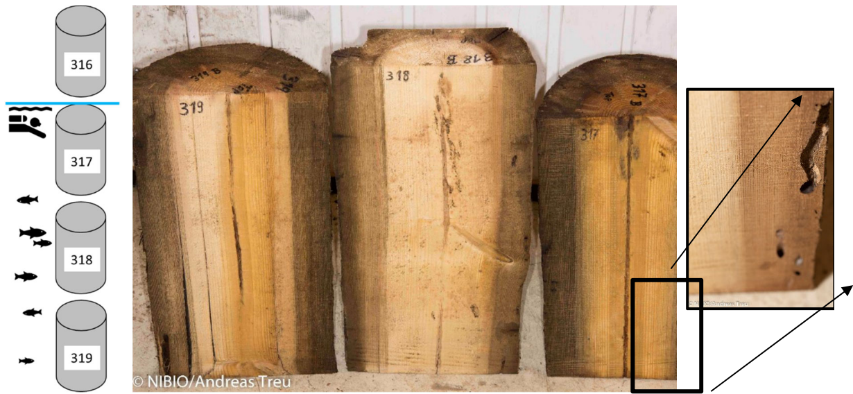
Figure 3. Borer attack of creosote treated wood pole removed from Hesselbergbrygga and close-up of borehole in creosote treated sapwood of Scots pine (right); drawing of position of pole segments in the water (left)
