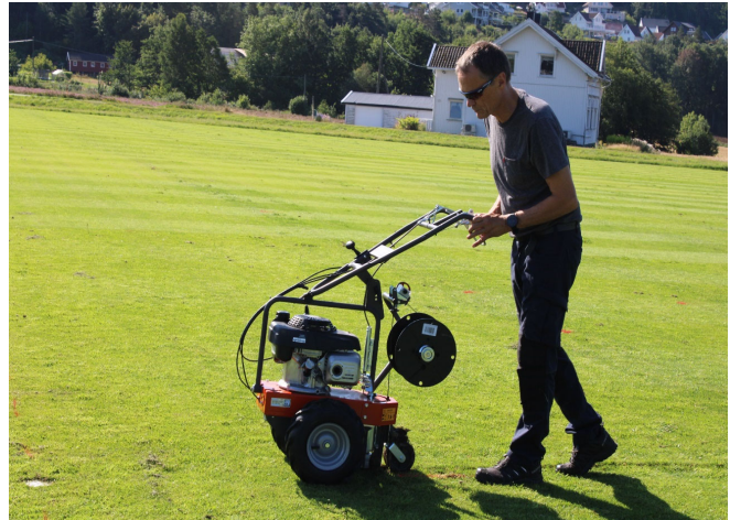
Photo 5. Installation of demarcation cables at approximately 5 cm depth around plots to be mown with a robotic mower. Photo: Karin J. Hesselsoe.
