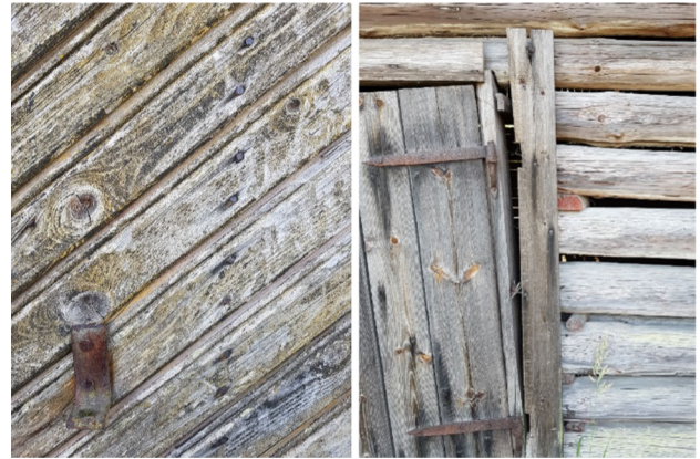
Figure 7 Examples of uncoated timber structures that have been exposed to the effects of weathering for near a century.
