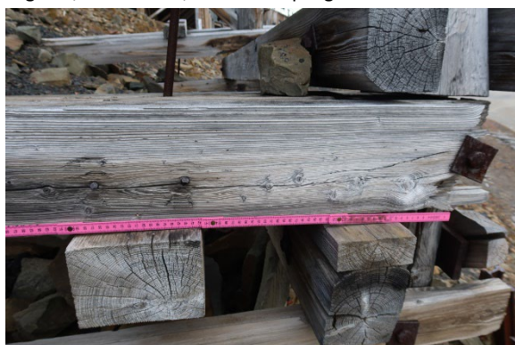
Leg NW, above ground, before sampling
