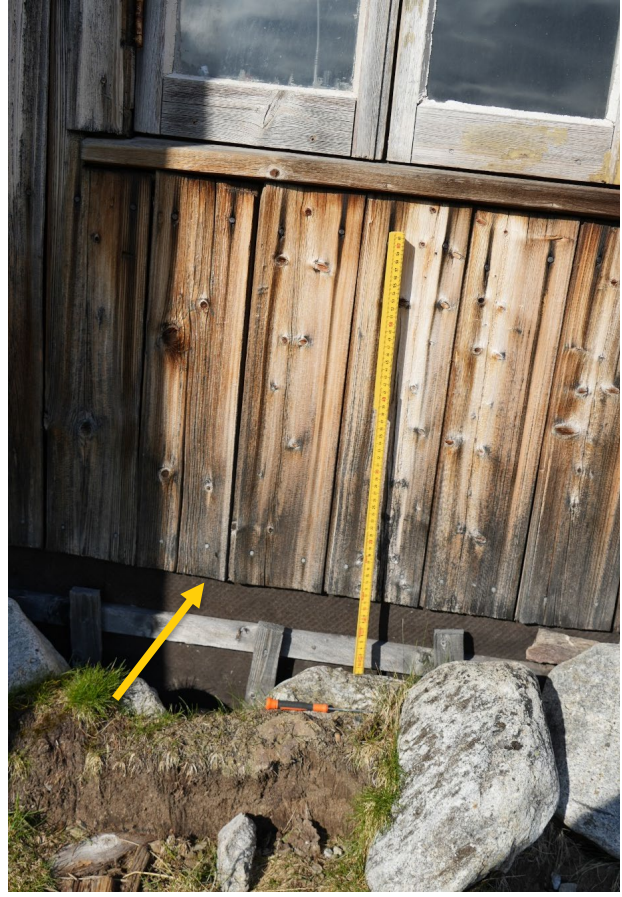
Camp Mansfield, façade facing west. Point of awl probing indicated. Awl probing performed on end grain of panel
