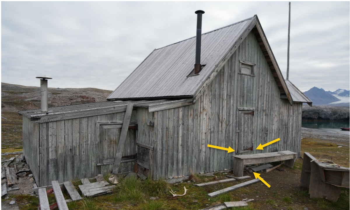
“Velferden”/Camp Lagercrantz, façade facing west. Points of awl probing indicated
