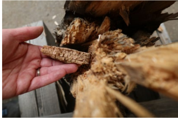
Cable car trestle 87889-16, object 2. Sample 2A9
