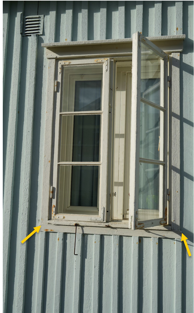
“Mexico”, façade facing south-west. Awl probing performed on end grain of weatherboard beneath window
