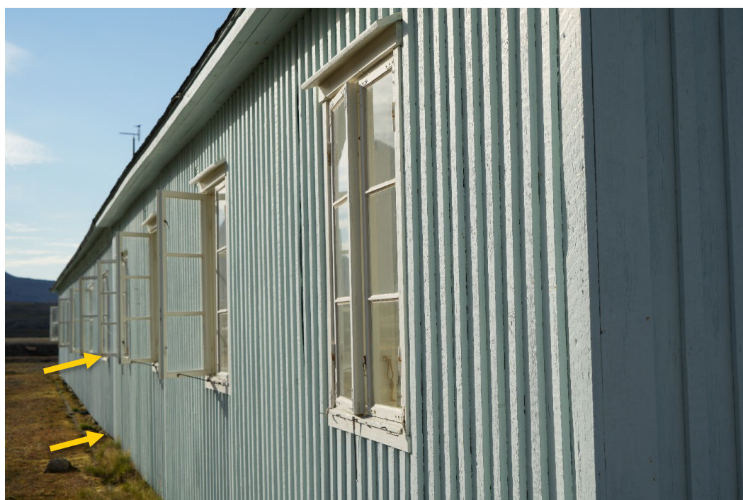
“Mexico”, façade facing south-west. Awl probing taken from window nr 4 from the corner, and from the panel underneath the window, next to the small stone.
