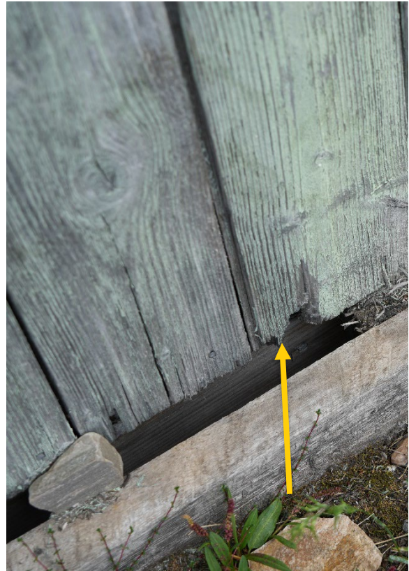
“Velferden”/Camp Lagercrantz, façade facing west. Point of awl probing indicated. Awl probing performed on end grain of panel
