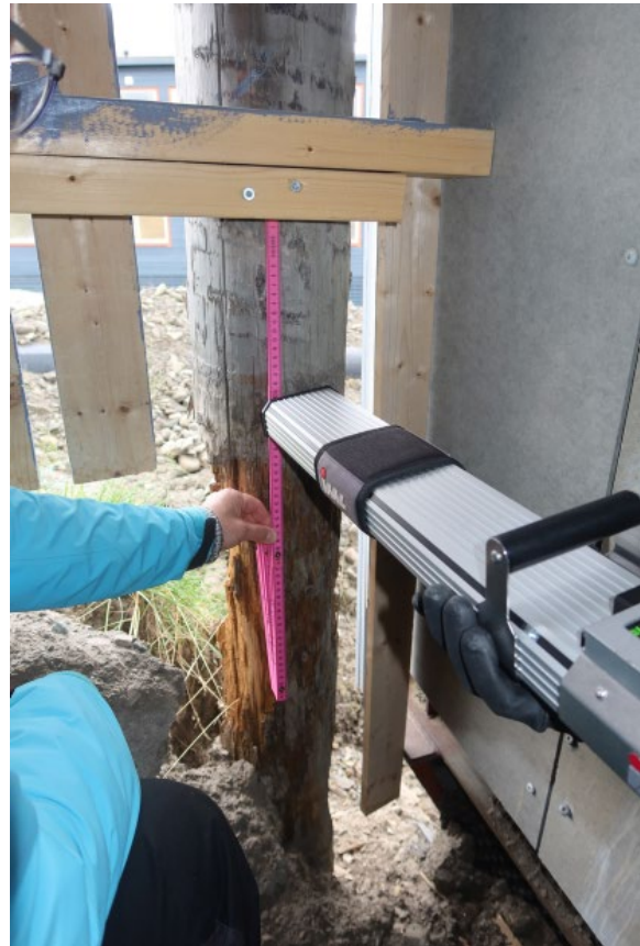
Hotel Radisson Blu, foundation pile SAS1. Decay detection drilling 233, 20 cm from beam
