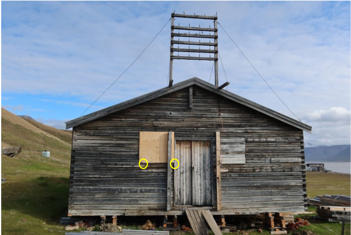
“Telegrafen”, overview west side. Awl probing points indicated
