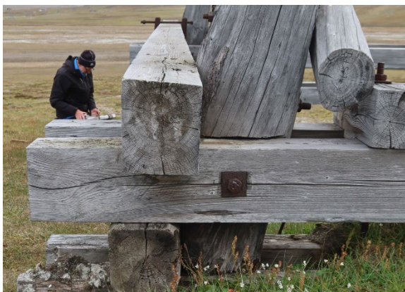
Leg NW, above ground, before sampling
