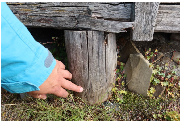
“Direktørboligen”, western facing side. Pile supporting bottom beam, before sampling. Point of drilling indicated
