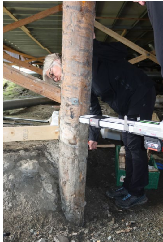
Hotel Radisson Blu, foundation pile SAS2. Decay detection drilling 244, cutting of sample SAS2-2
