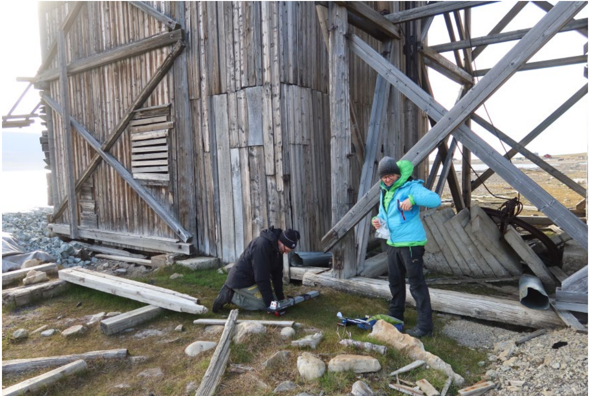
“Taubanestasjonen”, 93041-14. East side. Drilling, awl probing and sampling on beam beneath post, in the middle of the photo
