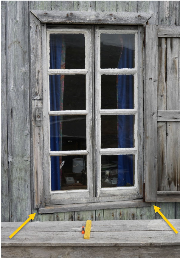
“Velferden”/Camp Lagercrantz, façade facing west. Point of awl probing indicated. Awl probing performed on end grain of weatherboard beneath window
