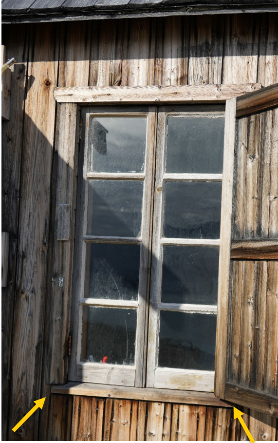
Camp Mansfield, façade facing south. Point of awl probing indicated. Awl probing performed on end grain of weatherboard beneath window
