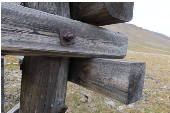
Leg NW, above ground, before sampling
