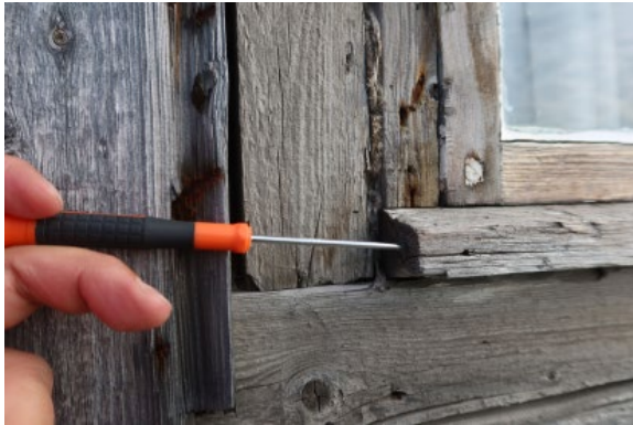
“Direktørboligen”, western facing side. Awl probing performed on end grain of weatherboard beneath main window
