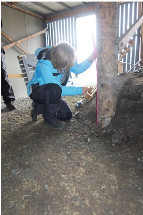
Hotel Radisson Blu, foundation pile SAS2. Probing with awl 40 cm from soil
