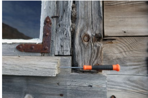
“Boligbrakke”, western facing side. Awl probing performed on end grain of weatherboard beneath southern window
