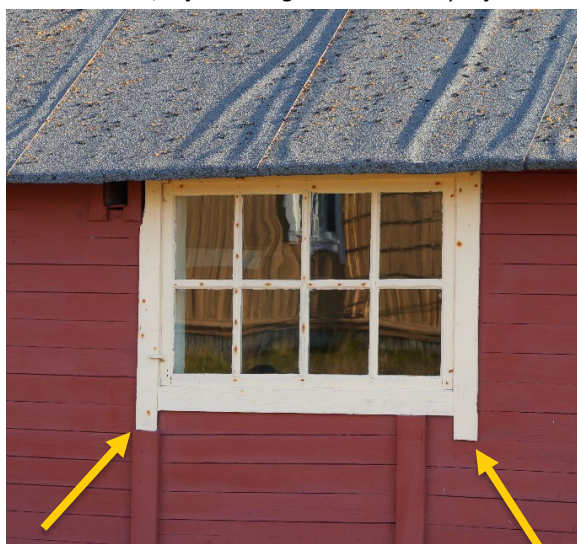
Green Harbour, window on façade facing north-east. Point of awl probing indicated. Awl probing performed on end grain towards north-west of weatherboard aside window
