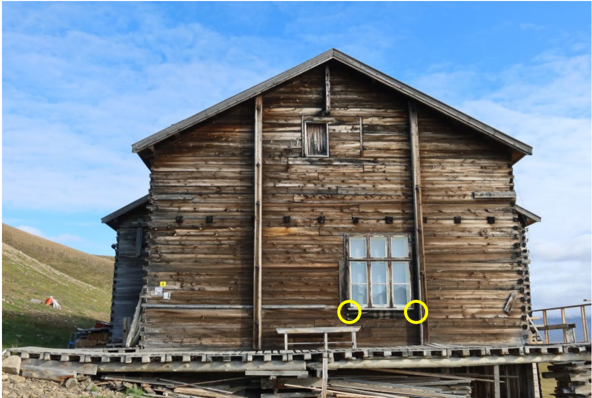
“Gamlemessa”, overview of façade facing west. Points of awl probing indicated
