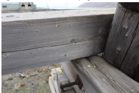
Leg NW, above ground, before sampling
