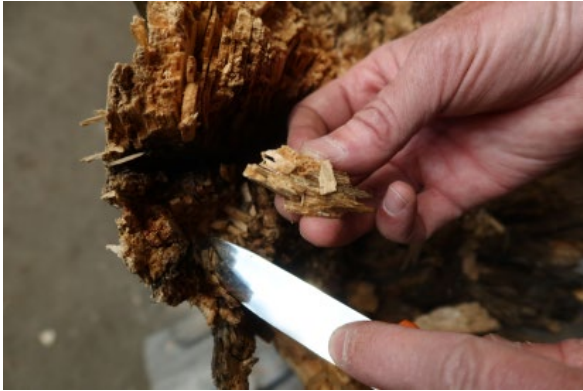
Cable car trestle 87889-16, object 1. Sample 1A7
