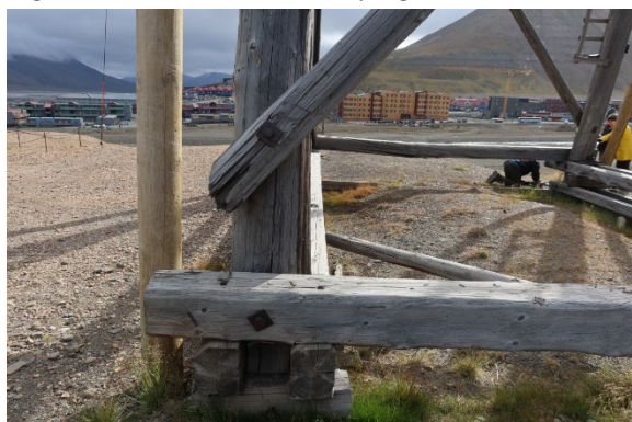
Leg NW, above ground, before sampling
