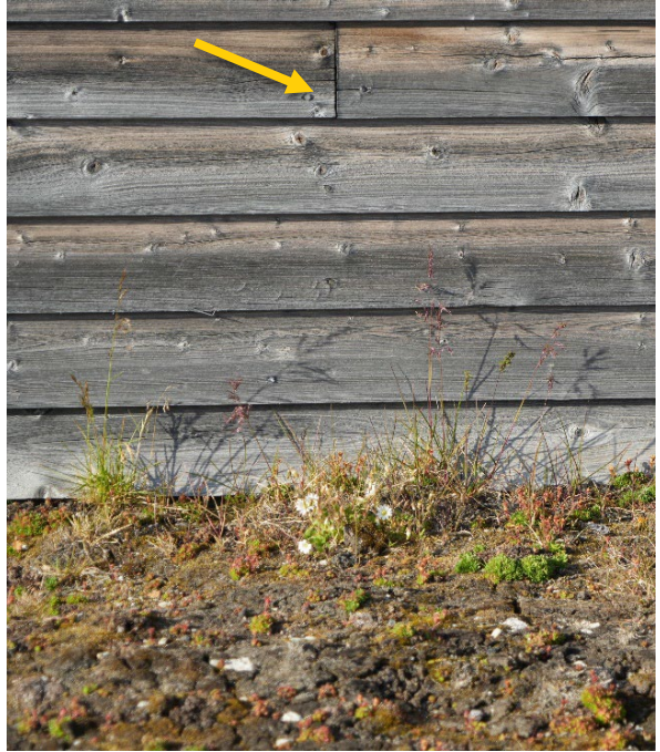
“Sætra”, south-west facing side. Awl probing performed on end grain of panel board beneath window.
