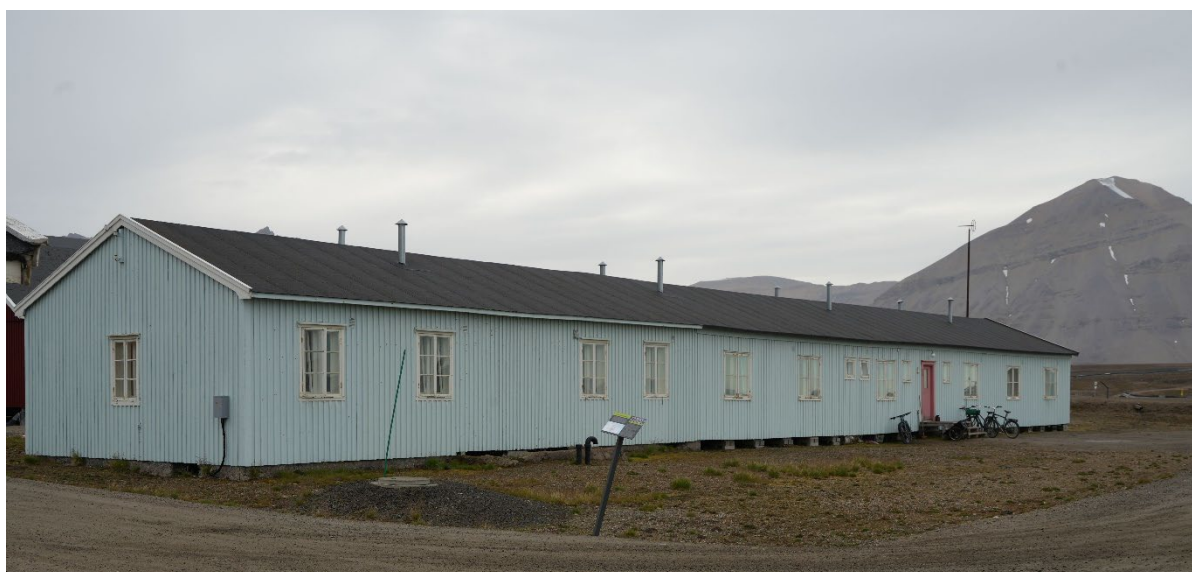
“Mexico”, façade facing north-east. Awl probing taken from the façade facing south-west.
