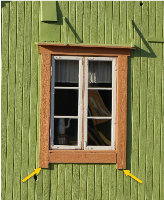
“Museumshytta”, façade facing south-west. Points of awl probing indicated. Awl probing performed on end grain of weatherboards aside window
