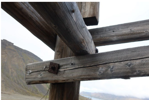
Leg NW, above ground, before sampling
