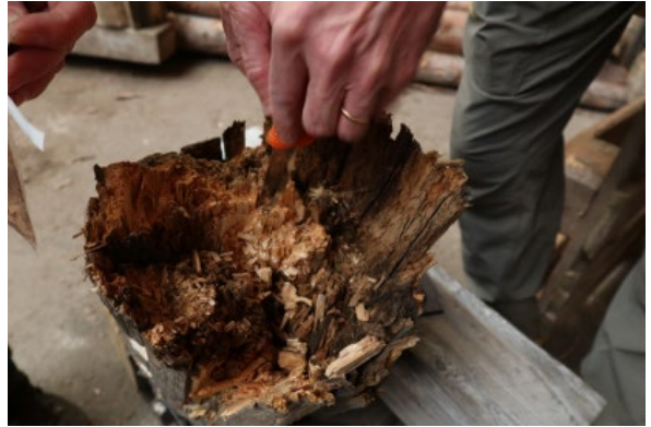
Cable car trestle 87889-16, object 1. Sample 1A8
