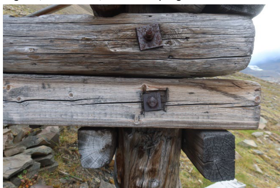
Leg NW, above ground, before sampling
