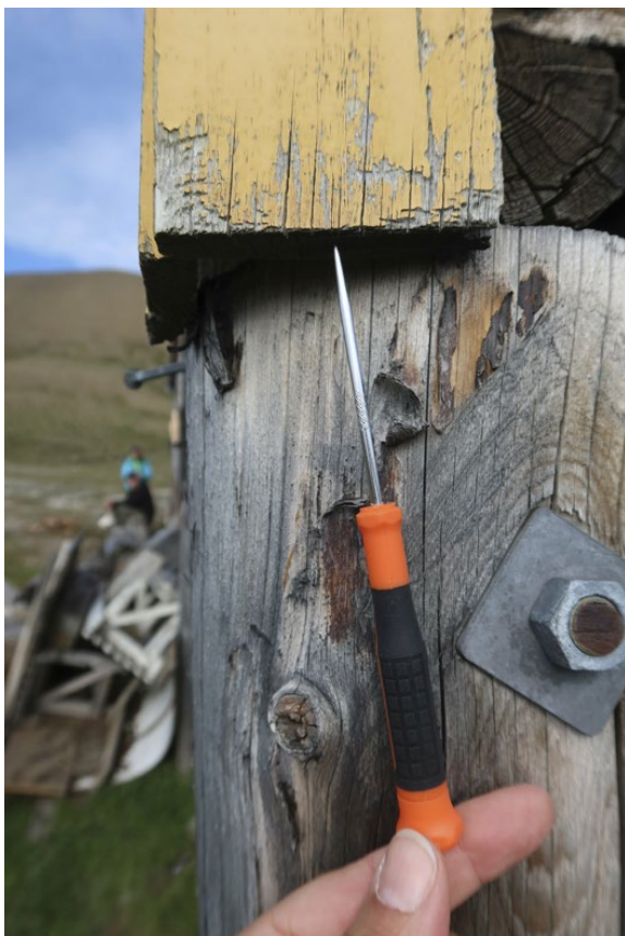
“Direktørboligen”, southwest corner. Awl probing performed on end grain of boards covering the corner
