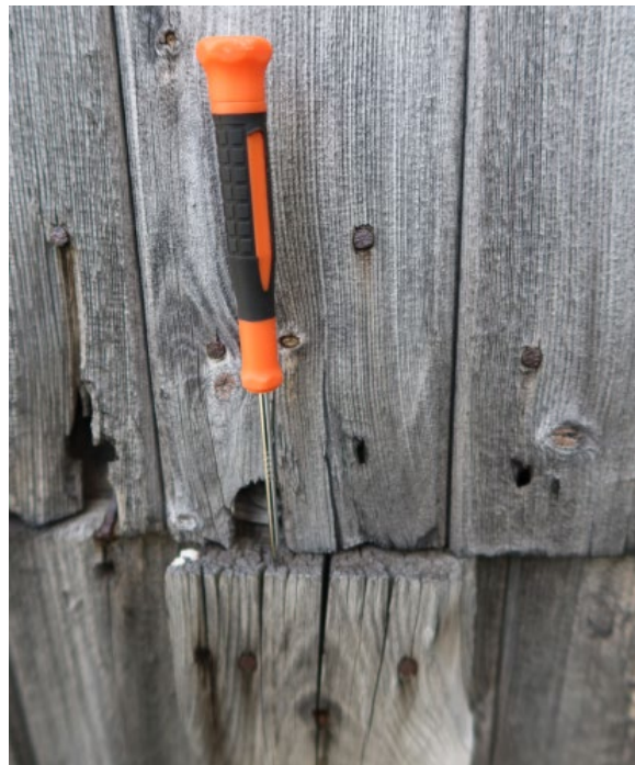
“Boligbrakke”, western facing side of covered porch. Awl probing performed on end grain of protruding board
