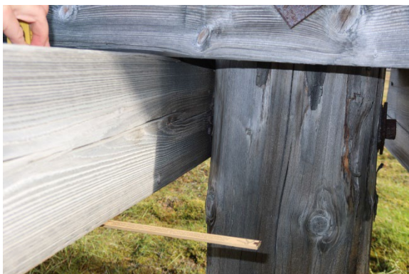
Leg NW, above ground, before sampling
