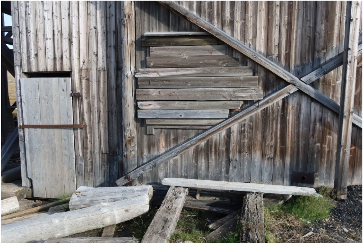
"Taubanestasjonen", 93041-14. West side, awl probing in end grain of boards covering window
