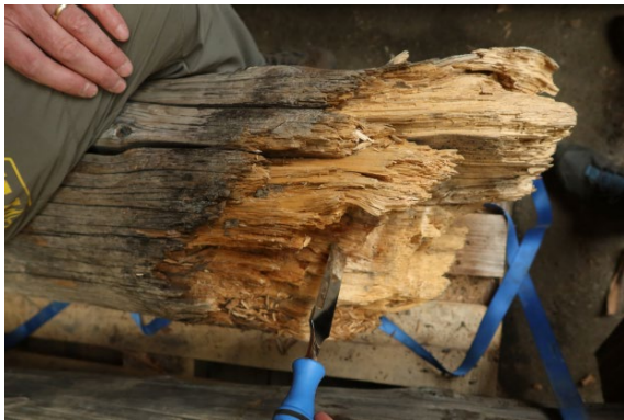
Cable car trestle 87889-16, object 3. Cutting of sample 3A12
