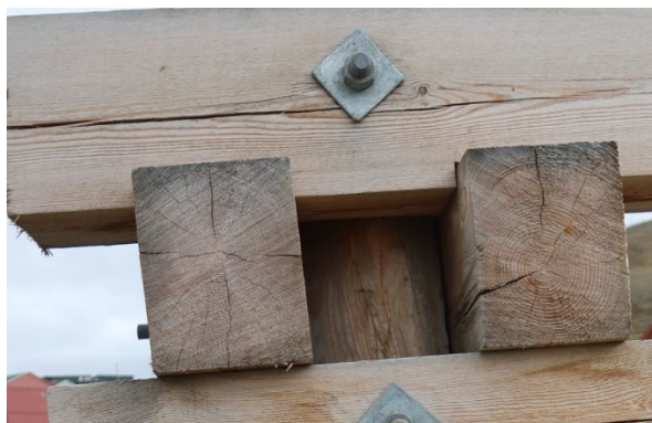
Leg NW, above ground, before sampling
