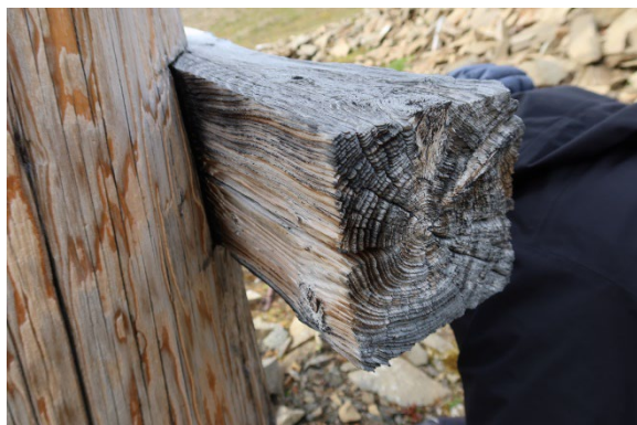
Leg NW, above ground, before sampling
