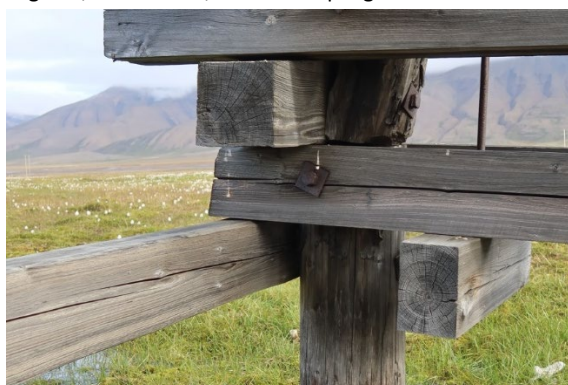
Leg NW, above ground, before sampling
