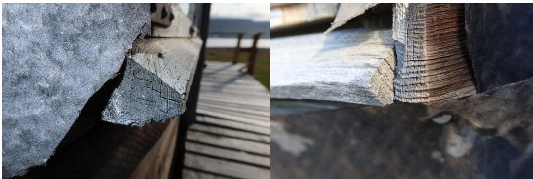
“Gamlemessa”, western facing window. Awl probing in end grain of weatherboard below window
