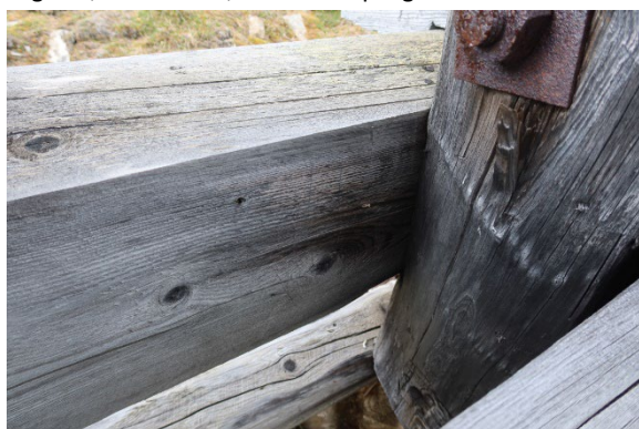
Leg NW, above ground, before sampling
