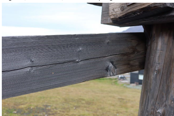
Leg NW, above ground, before sampling
