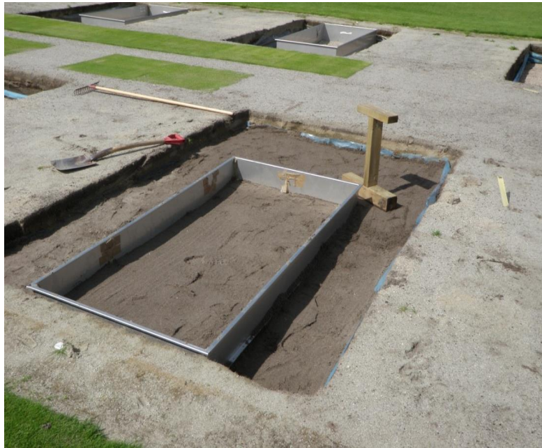
Photo 1: One of the lysimeters during construction in August 2011. The old rootzone was removed down to the gravel layer and USGA-spec. sand amended with either peat or compost was added. The lysimeters were 40-45 cm deep with a drain pipe located in the middle and a 10-15 cm gravel layer.
