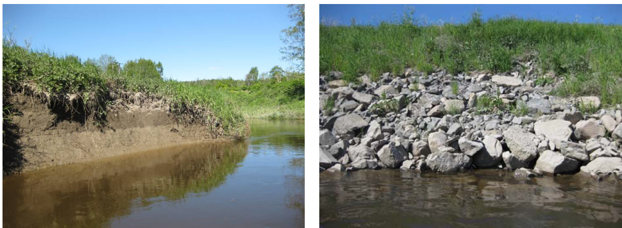
Figure 8. The erosion in River Hobølrelva is rather large (left) and erosion protection works have therefore been implemented in 2010 (right). Photos: E. Skarbøvik.
