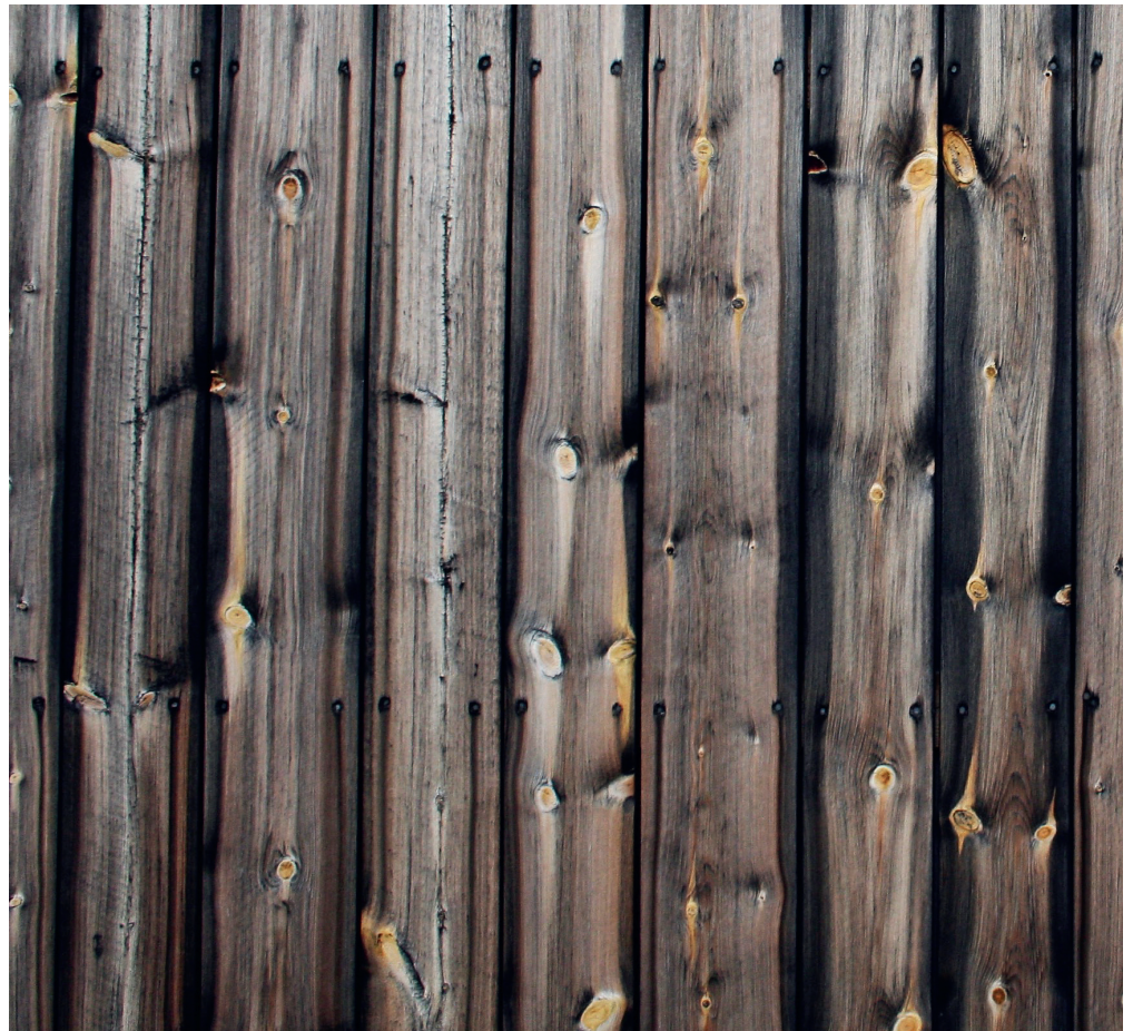
Run-off of rusty water on a Scots pine heartwood cladding.
