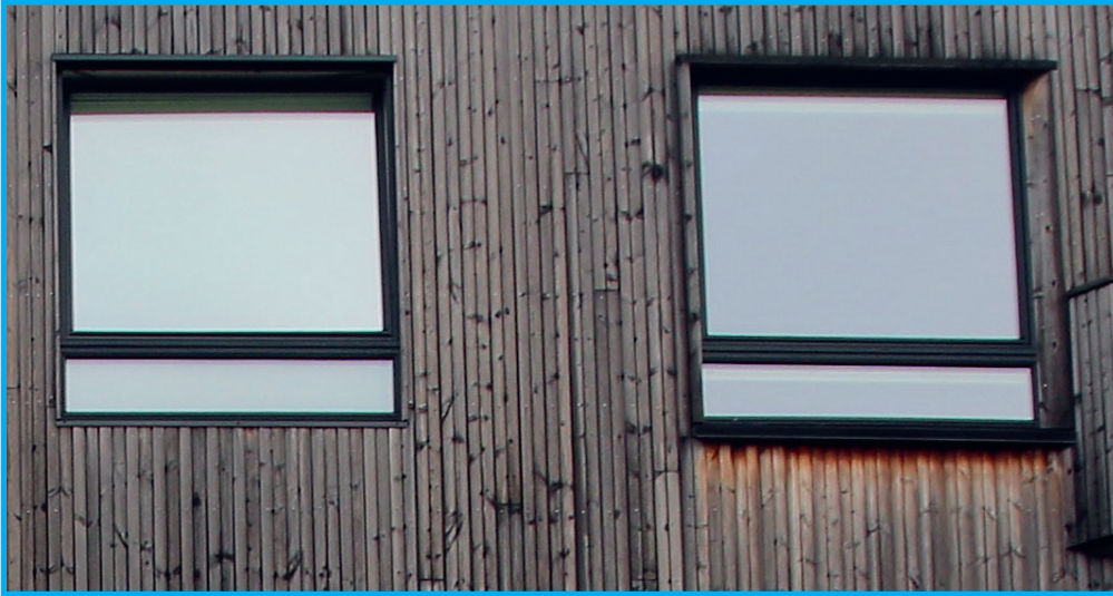
Cropped image 2. Window with narrow trims on the left. Projecting window trims on the right.
