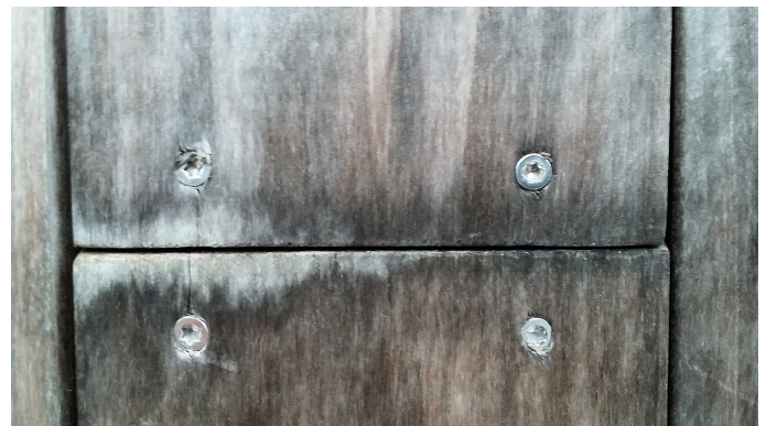
Small distance between cladding boards.
