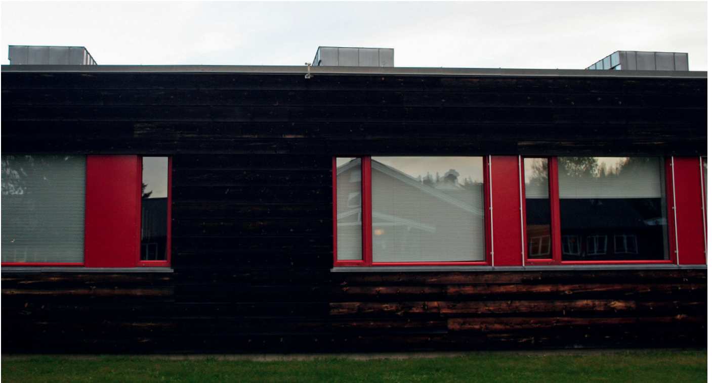
Wet south-facing façade. Lecture building, Sessvollmoen Military Camp.
