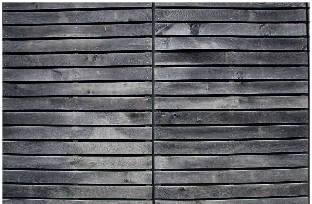
Horizontal, open aspen cladding including a great amount of warped boards.
