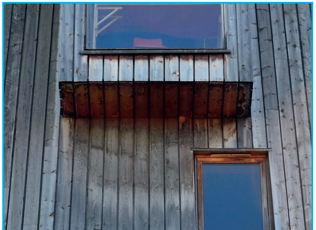
Visible water accumulation under an oriel.
