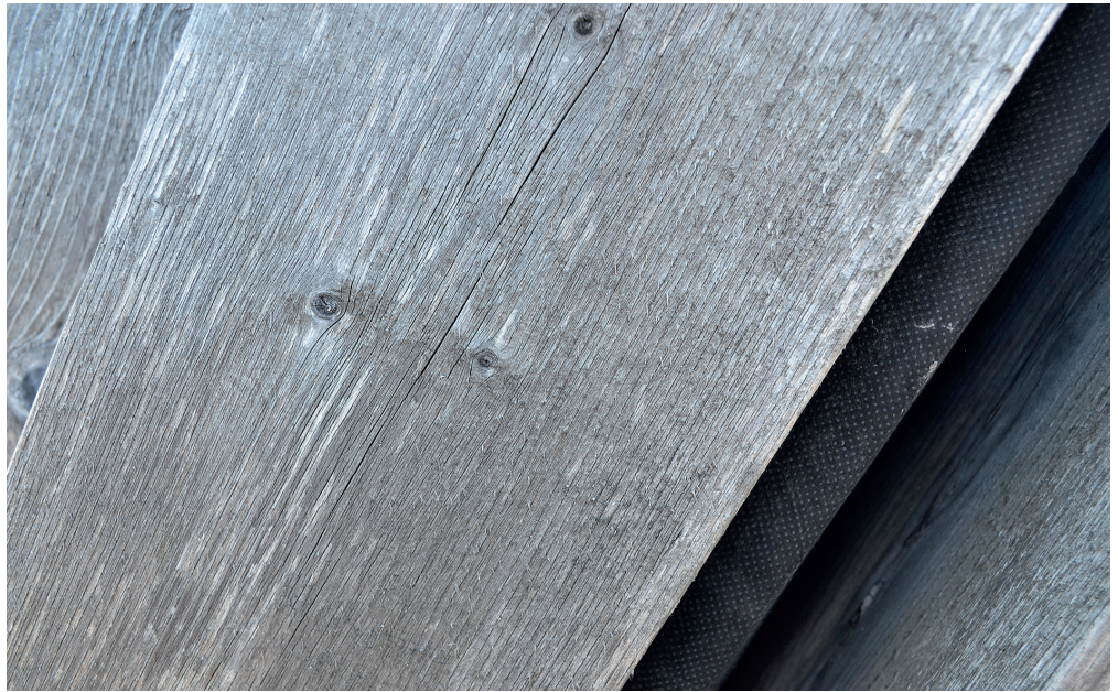
Fibrous surface of a cladding board
