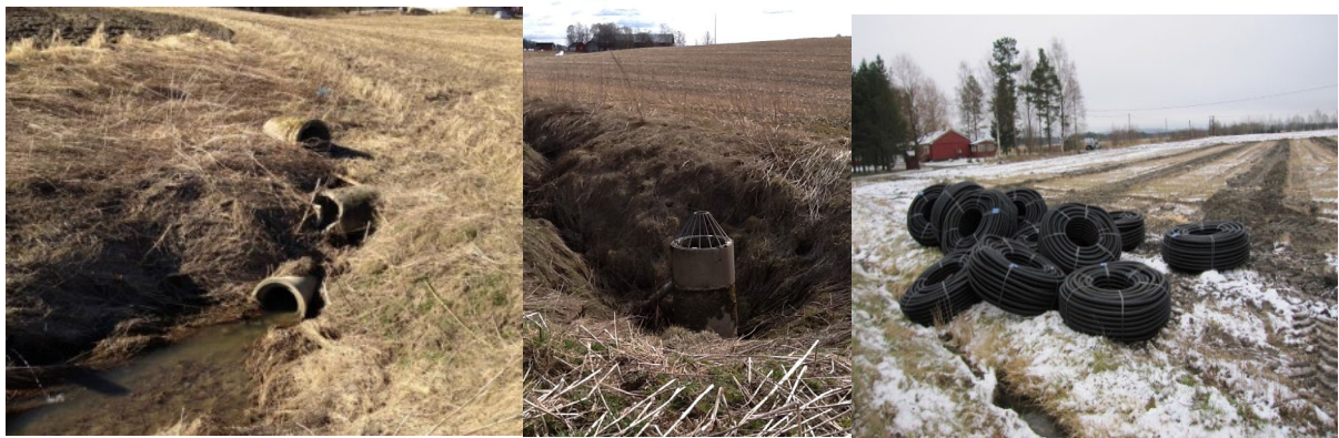
Figure 3.4. Repair of damaged drainage systems and inlets for surface runoff (Photos: Atle Hauge, Lillian Øygarden)
